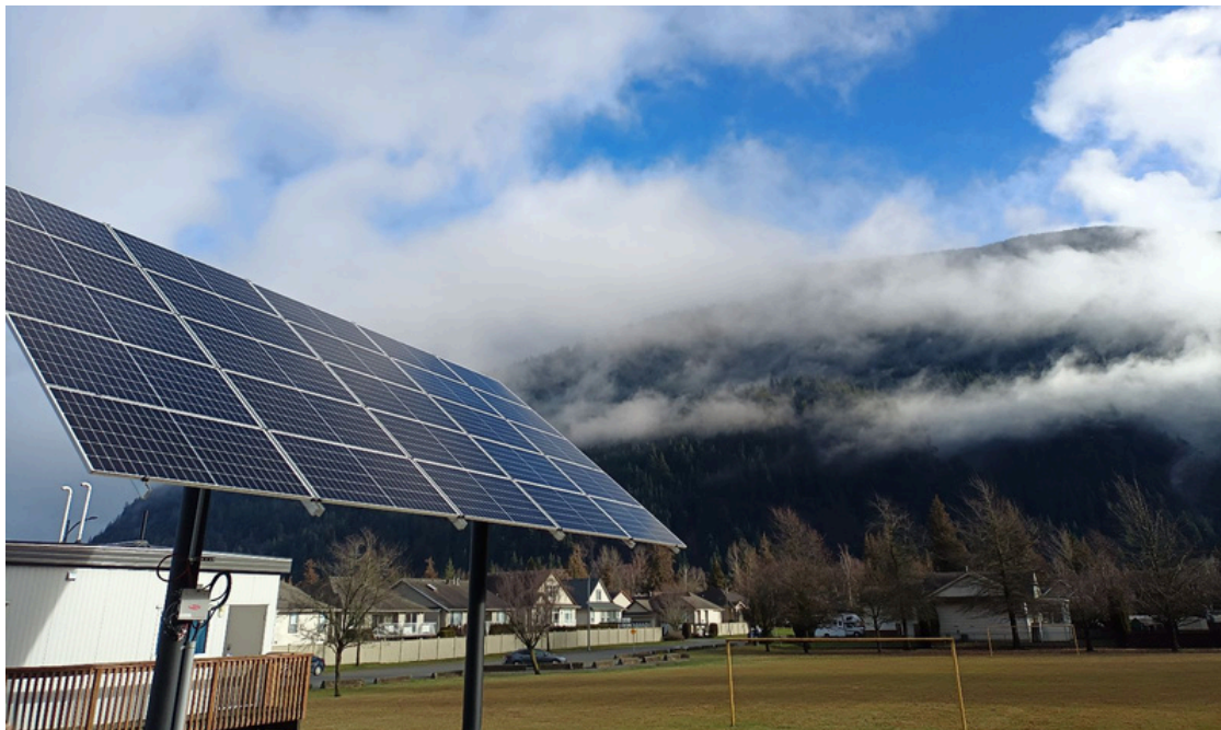
Solar installation in Hope, British Columbia
