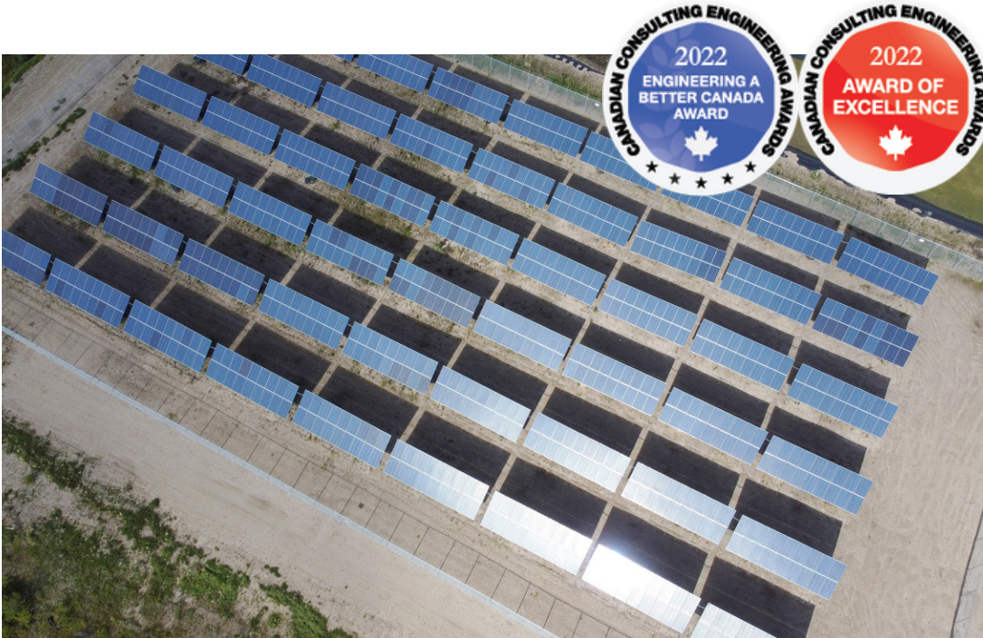
Fort Severn Solar Array in Northern Ontario.
