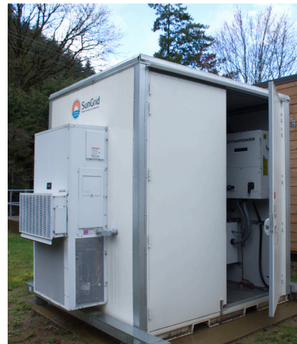
Battery storage system.
